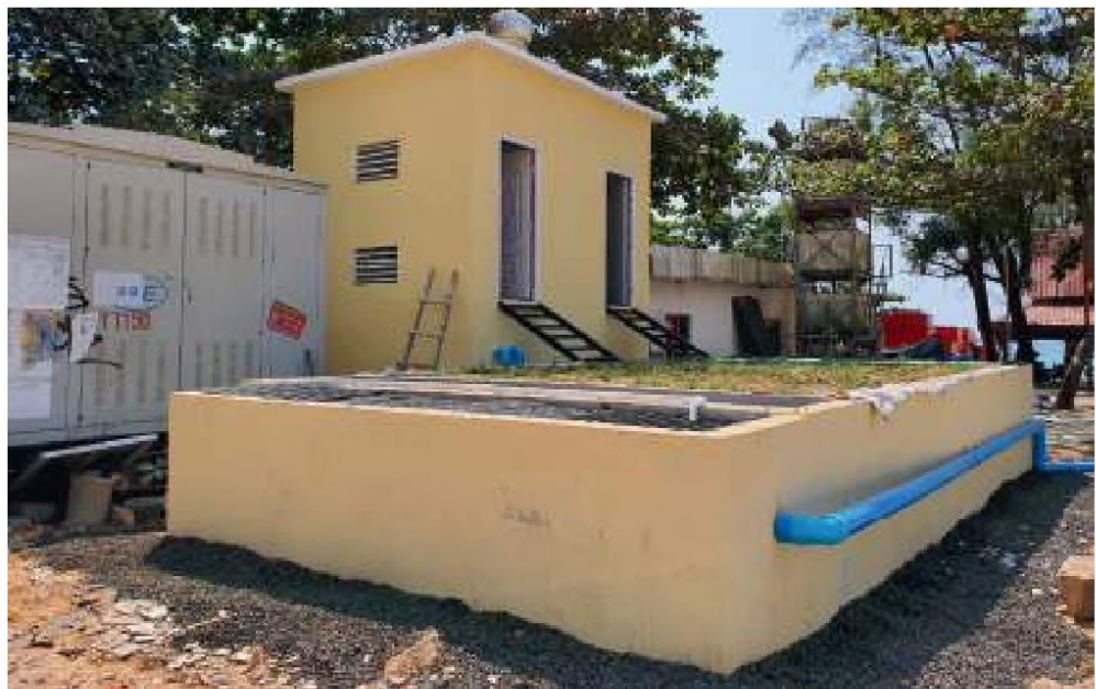
Angular View of Wastewater Treatment System_A
