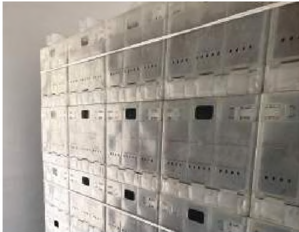
View of Bio-Filtration
