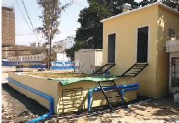
Angular View of Wastewater Treatment System_B
